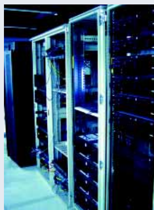
托管的主要设备 Primary equipment of Data Warehouse
